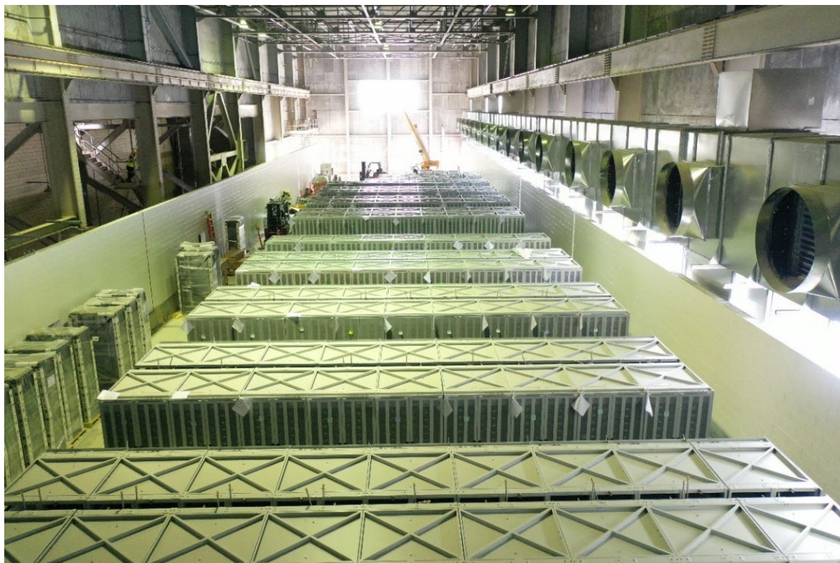
Picture 2: Moss Landing Battery – Phase 1 Facility
