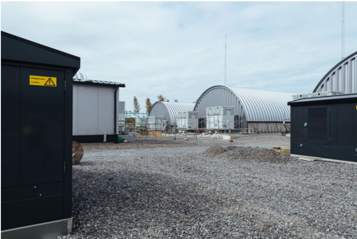
Picture 4: Olkiluoto Battery
